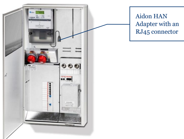
Figure 2: Example installation of the HAN adapter solution.
